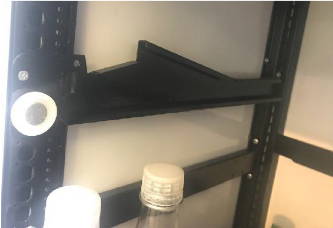
Tray sliders and mounting holes in cabinet
